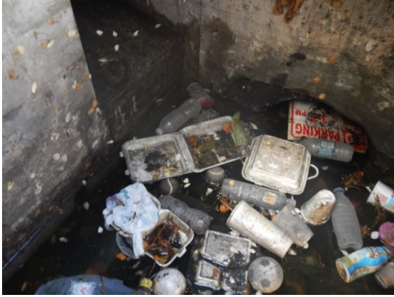
Catch basin full of trash in Honolulu
