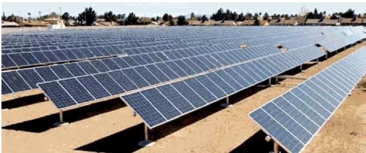
Figure 6: An example of ground-mounted solar panels with trackers to adjust the angle to maximize sun exposure.
