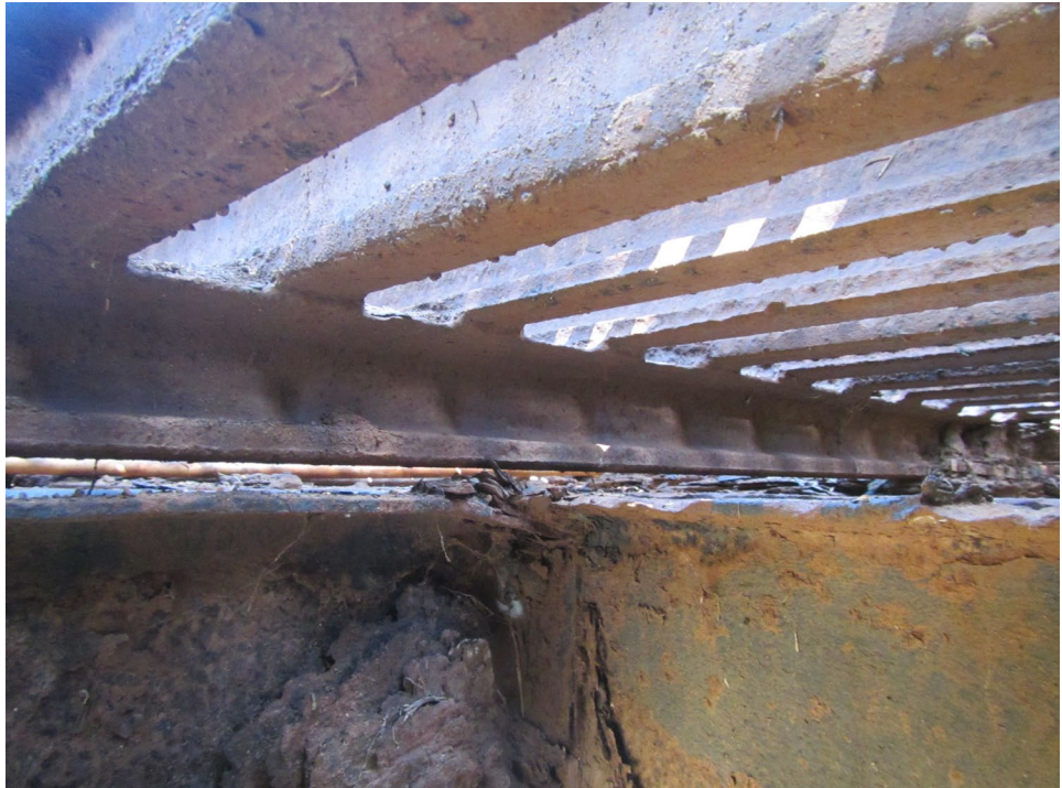
Photo 7 – Gap Between Transverse Rail and Corroded Girder Below
