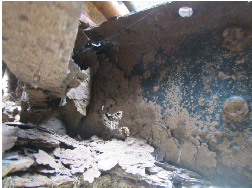
Photo 8 – Severe Through Corrosion at Perimeter Channel Girder Web
