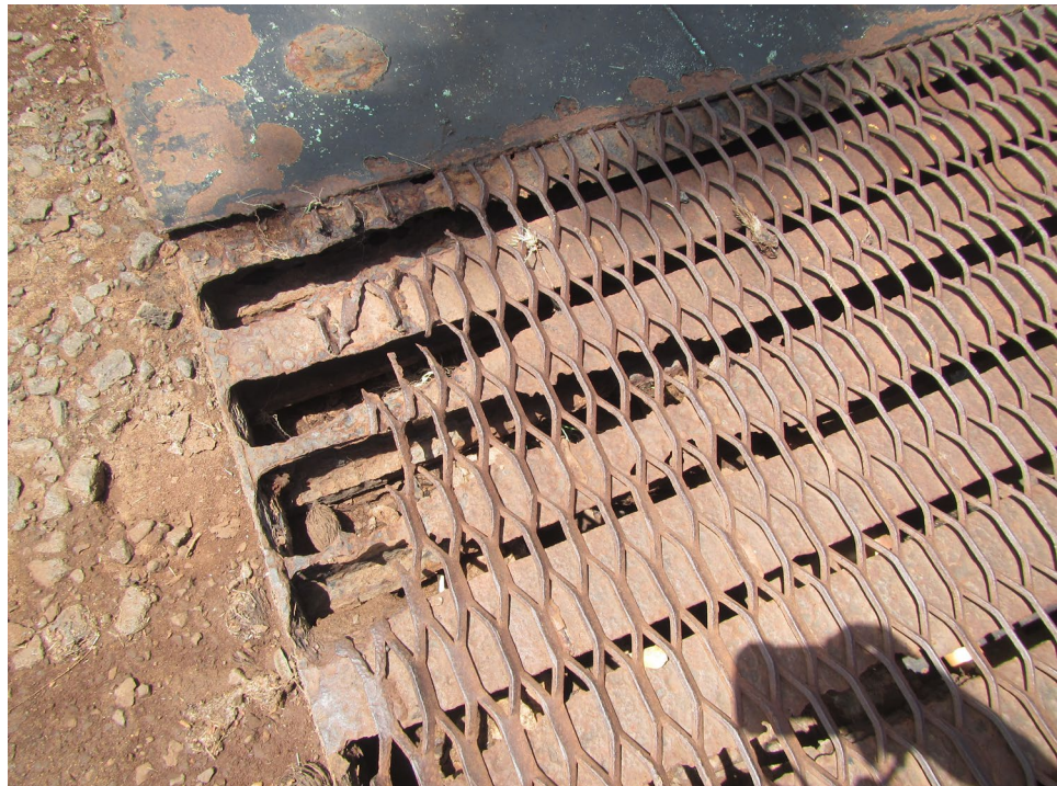
Photo 6 – Severe Corrosion and Depression in Top Rails
