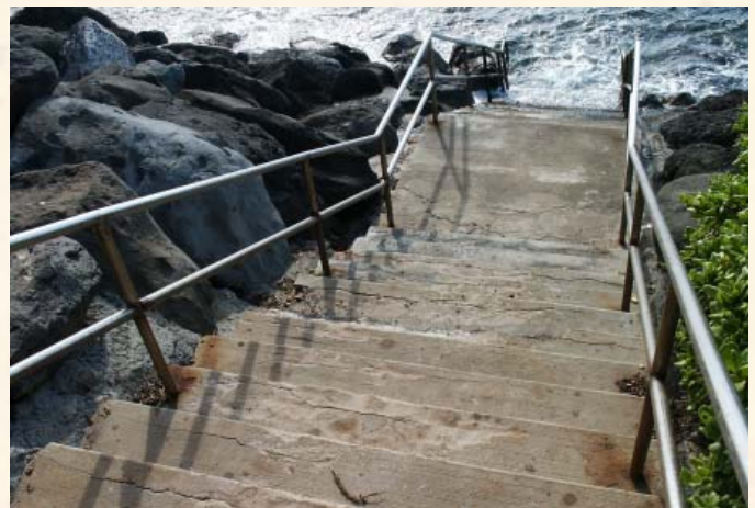
Deteriorated hardscapes, fixtures & furniture in the Kaka'ako Parks will be repaired.
