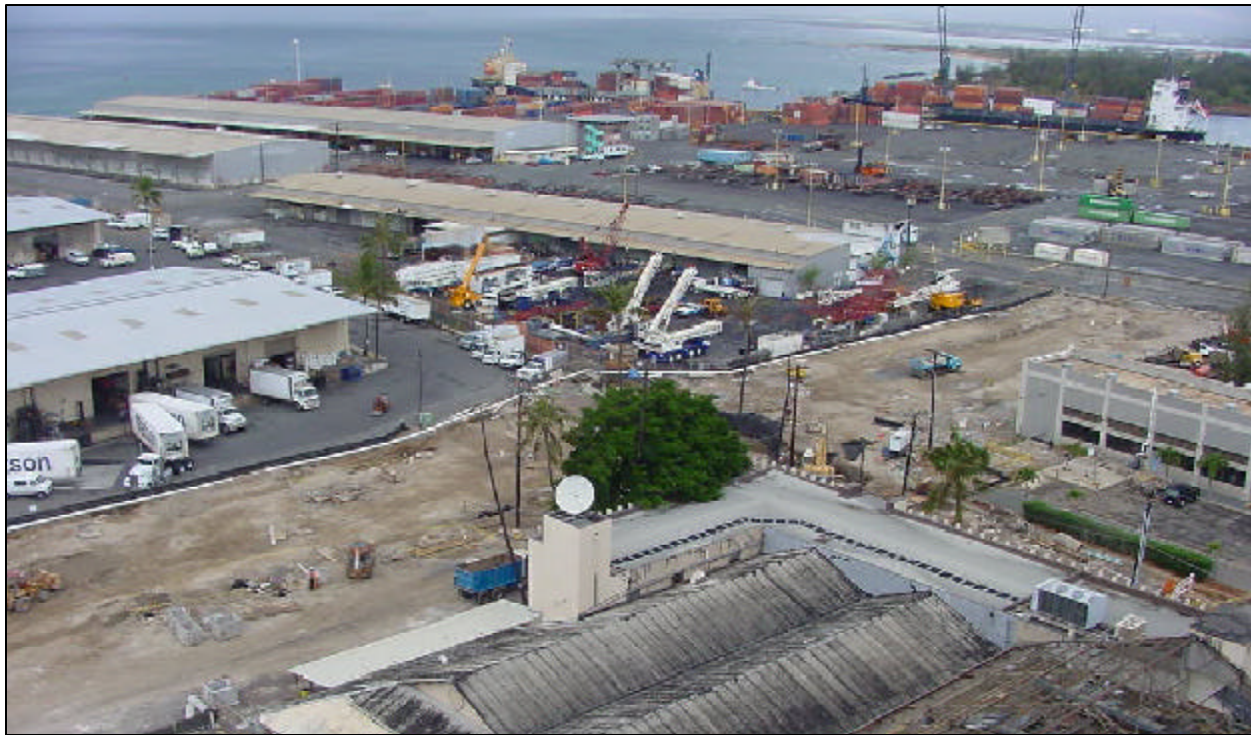
Ilalo Street improvements extended from Ahui Street to Forrest Avenue (South Street).
