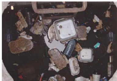
Litter found inside a Kakaako catch basin
