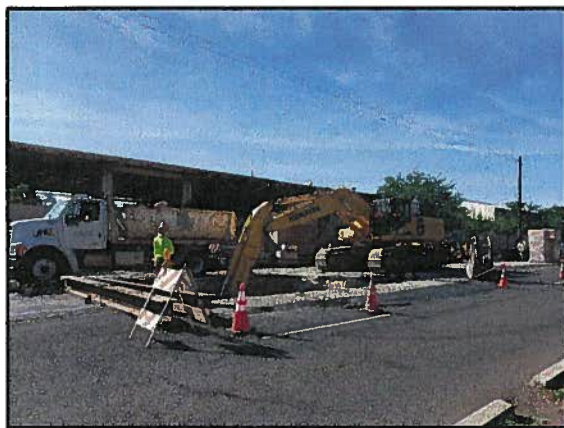
Paul's Electric begins manhole installation fronting the Hawaii Army National Guard on Enterprise Avenue.
