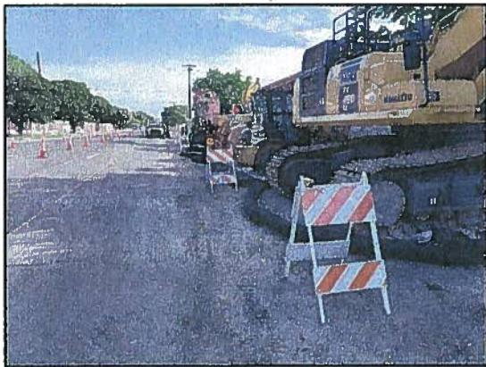
Paul's Electric completes manhole installation fronting the Hawaii Army National Guard on Enterprise Avenue.
