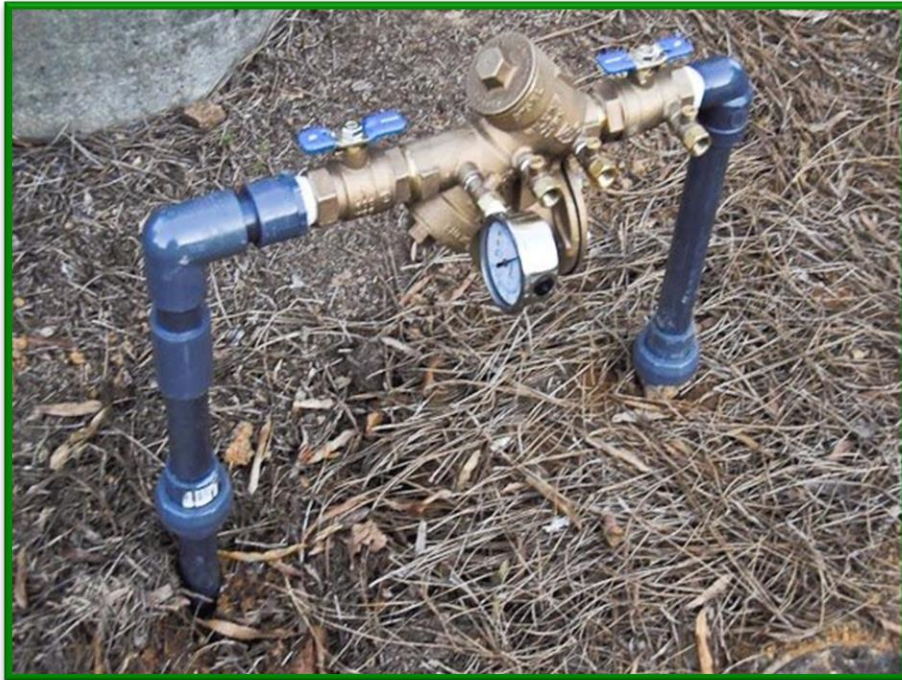
Figure 28: Example of Irrigation Backflow Preventer
