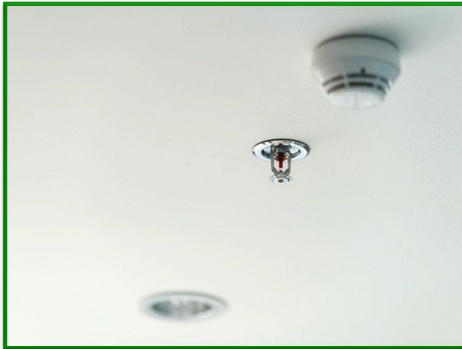
Figure 22: Example of Interior Fire Sprinkler and Alarm System
