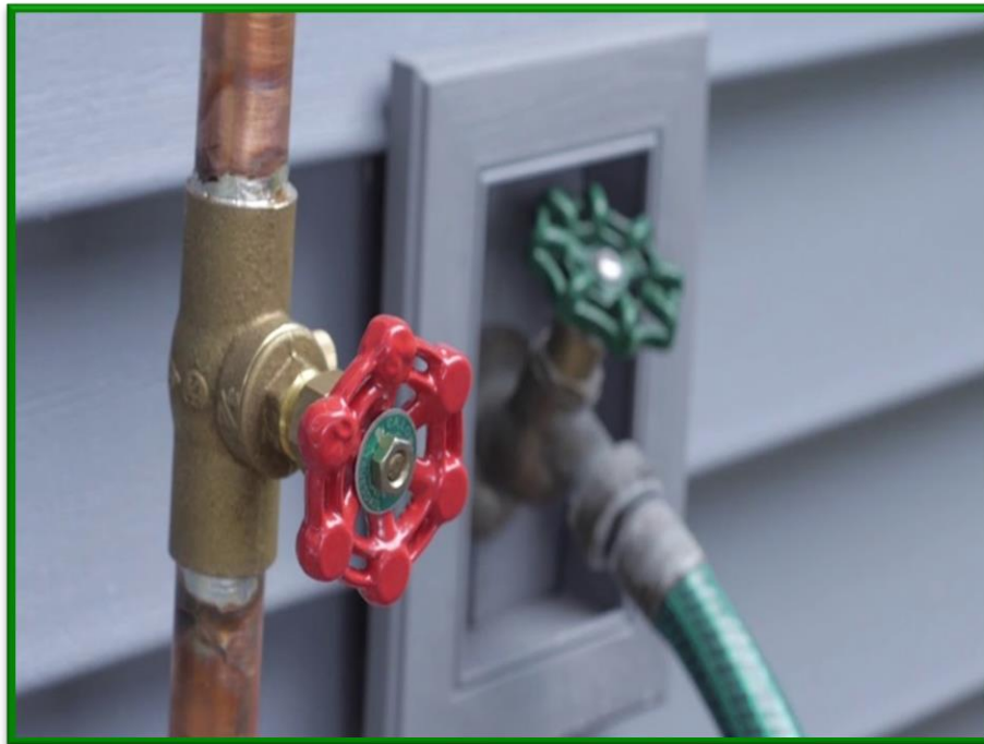
Figure 30: Example of Water Shut-Off Valve
