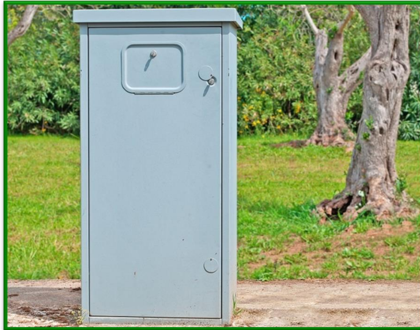
Figure 13: Example of an Outdoor Electrical Control Panel
