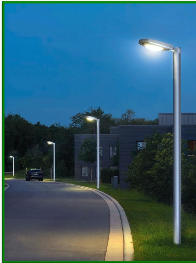
Figure 14: Common Area Lighting Pole Example
