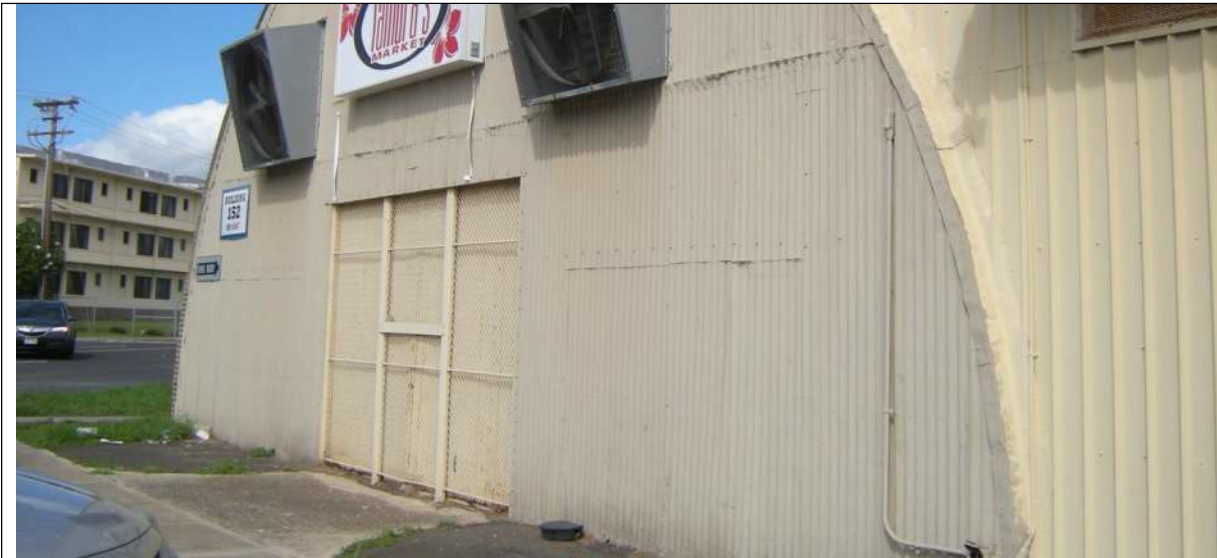
Fig. 5. (2014 Appearance.) View of large-scale opening in 2014 that has since been expanded in height. The door shown here that was later removed and replaced was likely in place since the 1960s.
