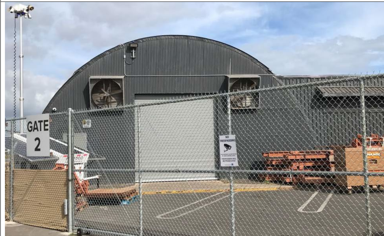
Fig. 6. (2021 Appearance.) View of Enterprise Avenue façade in 2021 showing fenced enclosure and the replacement (roll-up) door changes made in Phase 2. New door is taller in height than the historic period.
