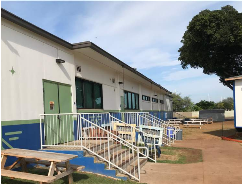
Fig. 6 (2021 Appearance) South side view. New doors, windows, and handrails have been installed. Windows and doors are for the most part in keeping with the original fenestration pattern and openings, however one window opening was infilled. The blue-tinted glazing of the new windows is not historically appropriate. Original handrails have been removed and replaced. The historically inappropriate shade awning frames have been removed. Integrated gutters have been added at eaves, which was likely not original feature. Rain chains have been added at intervals, which are not historically appropriate.
