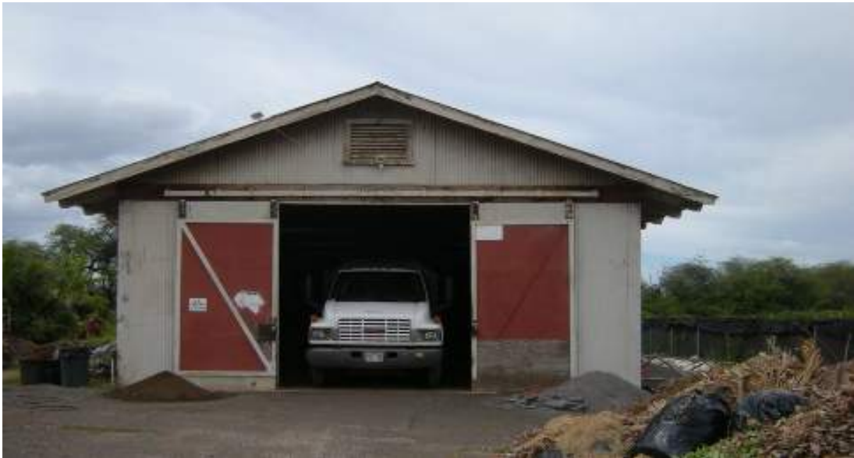
Fig. 1. Building 476, 2014 façade (view from Nassau Street). When MASON last surveyed this building in 2014, it was in poor condition, with extensive termite damage. The roof and siding material was corrugated metal.
