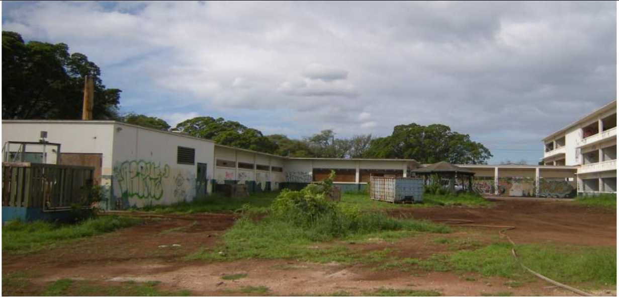
Fig. 8. (2014 Appearance.) Rear View, from within courtyard, with breezeway to former BOQ at right.
