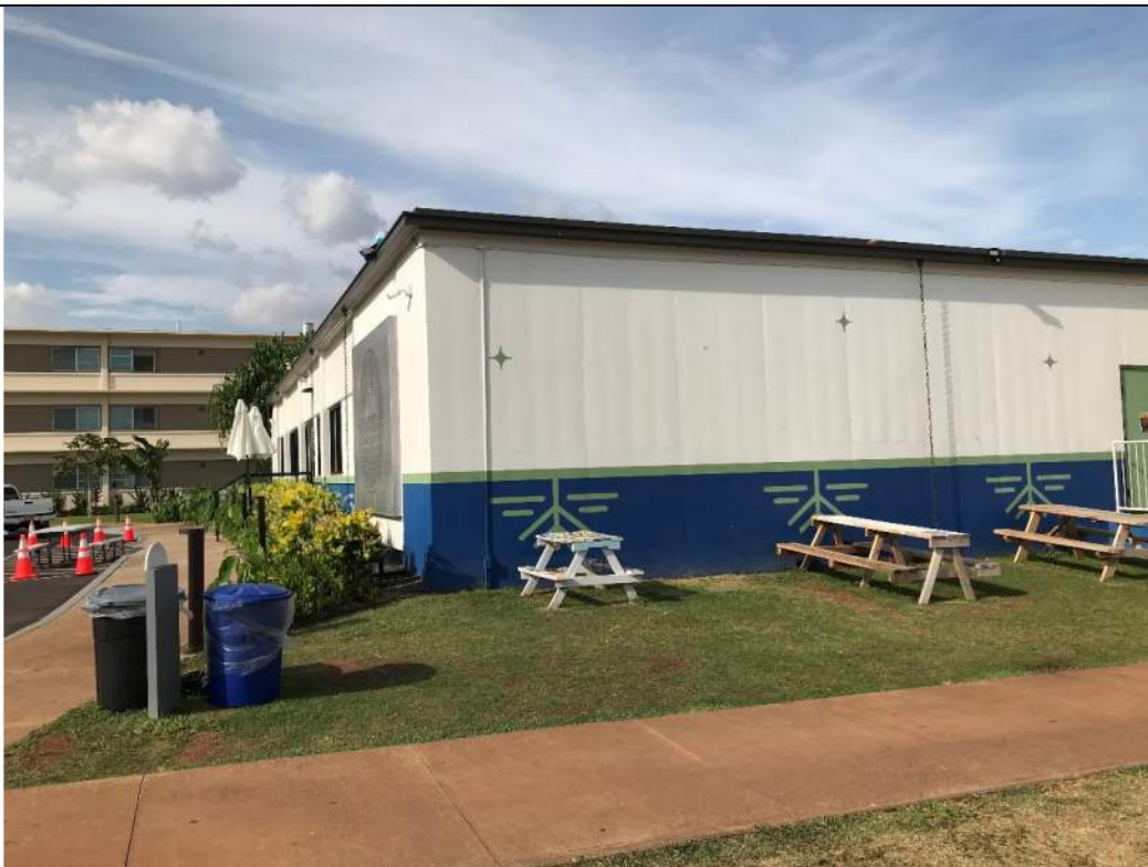
Fig. 4. (2021 Appearance.) Southwest corner. New gutters surround the building, with historically inappropriate rain chains at intervals.
