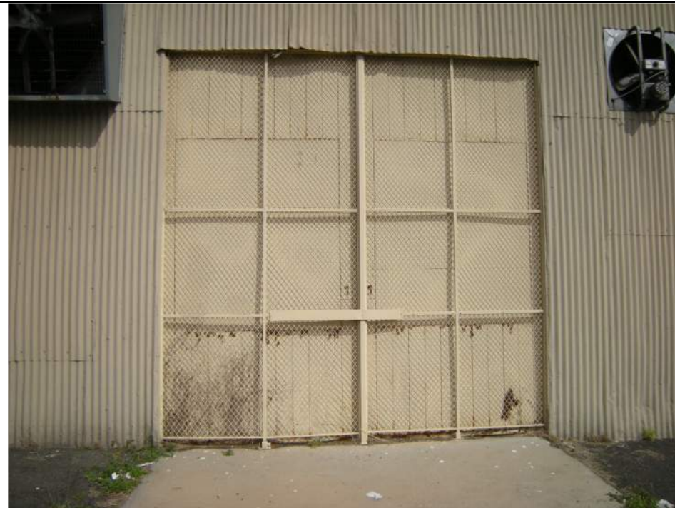
Fig. 5. (2014 Appearance.) Door on right side that has been replaced. Height has been retained. This door was likely in place since the 1960s. See drawing in Fig. 9.
