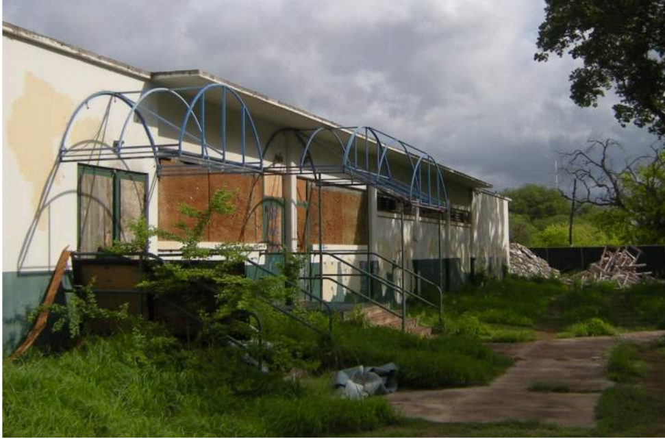
Fig. 5. (2014 Appearance.) South side view. Windows and doors were boarded up. Flashing had been stripped from the eaves. Remnants of historically inappropriate shade awnings were over windows and doors. Original stair rails were intact.
