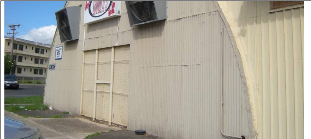
Fig. 3. (2014 Appearance.) View of large-scale opening in 2014 that has since been expanded in height. The door shown here that was later removed and replaced was likely in place since the 1960s.
