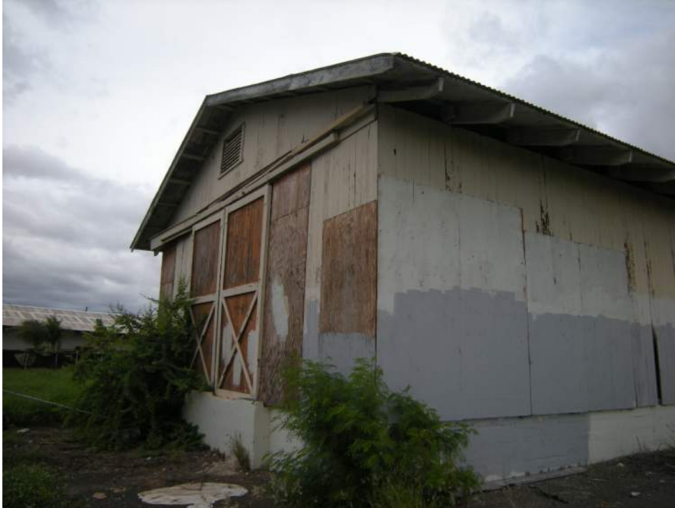
Fig. 9. Building 477, 2014 appearance of the rear, which faces Midway Avenue. Extensive termite damage had led to temporary plywood repairs.
