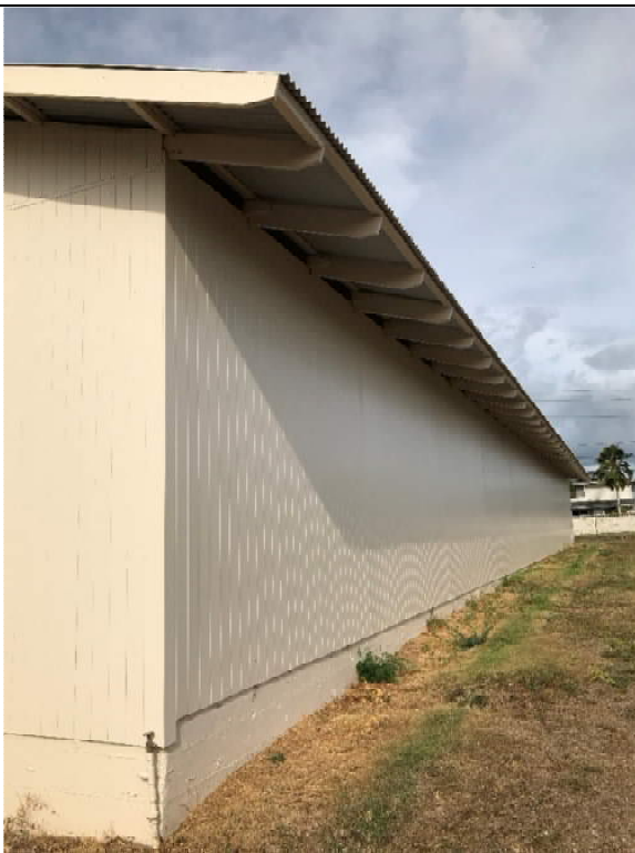
Fig. 4. Building 476, 2021 appearance of south side in 2021. The corrugated metal siding was replaced with wood siding, which is a historically appropriate material.
