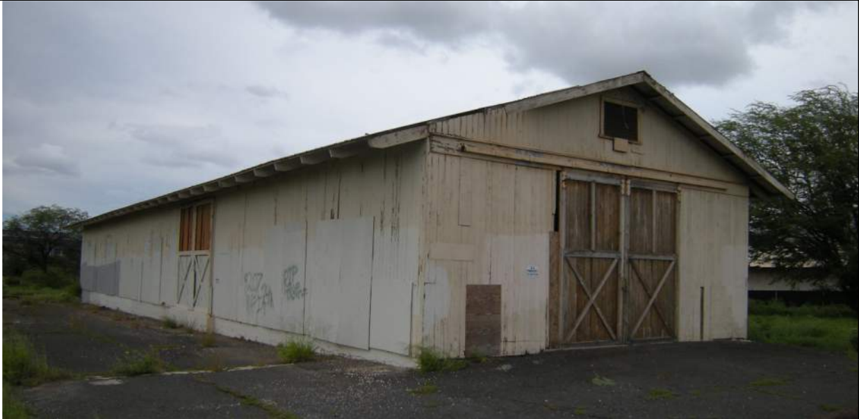
Fig. 7. Building 477, 2014 appearance. When MASON last surveyed this building in 2014, it was in very poor condition. It had extensive termite damage, with many sections of the building covered in plywood boards, and portion of the roof and eave on the Nassau (front) had collapsed. The building was sided with wood (unlike Building 476, which was originally sided with corrugated metal).
