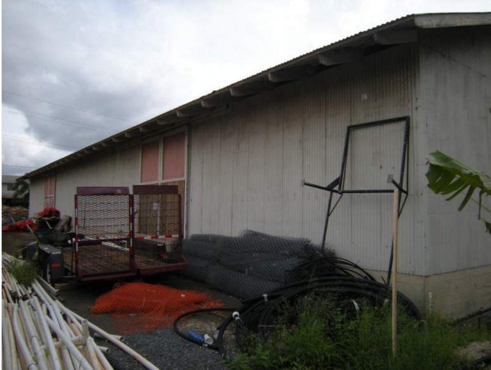
Fig. 5. Building 476, appearance of north side in 2014, showing two sets of large-scale sliding doors. The pair in the foreground had been partly boarded up with plywood to cover damaged wood.
