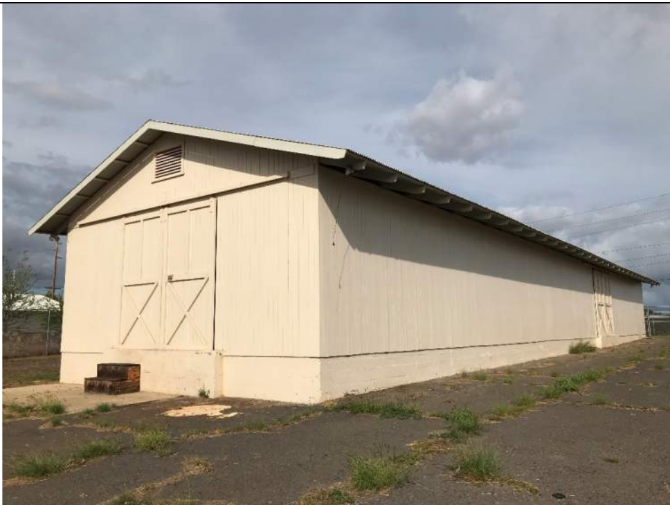
Fig. 10. Building 477, 2021 appearance of the rear, which faces Midway Avenue. Extensive in-kind repairs were made by Hunt to return the building to its previous appearance.
