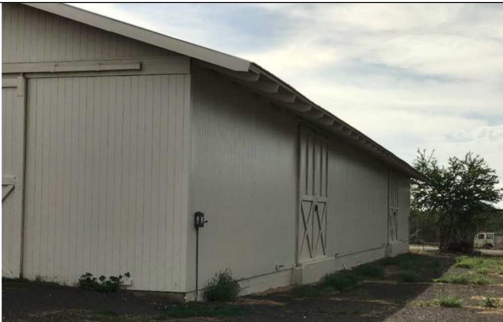
Fig. 6. Building 476, appearance of north side in 2021, showing two sets of large-scale sliding doors. The doors were repaired in an historically appropriate manner.
