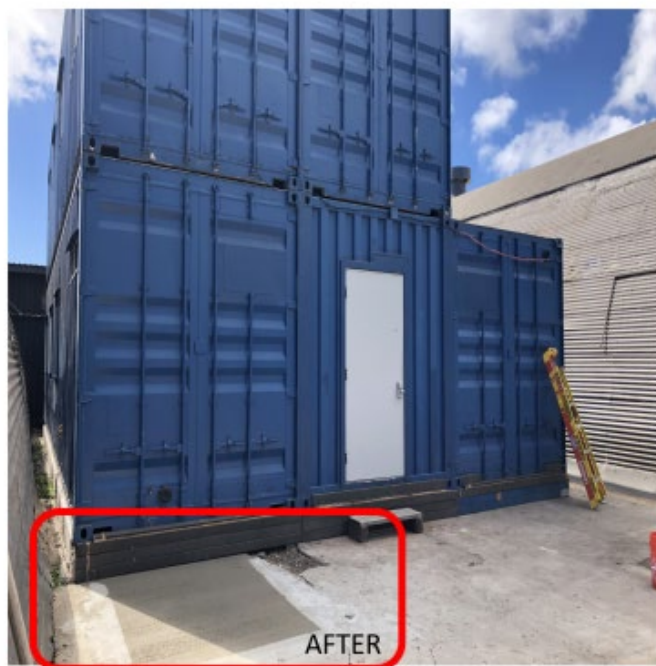
Figure 7 Swinerton removed the holding tank and infilled with concrete as part of an effort to restore the area to its original condition.
