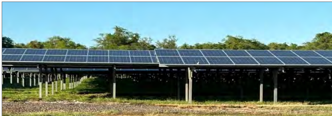
The 5-megawatt Aloha Solar Energy fund solar facility
