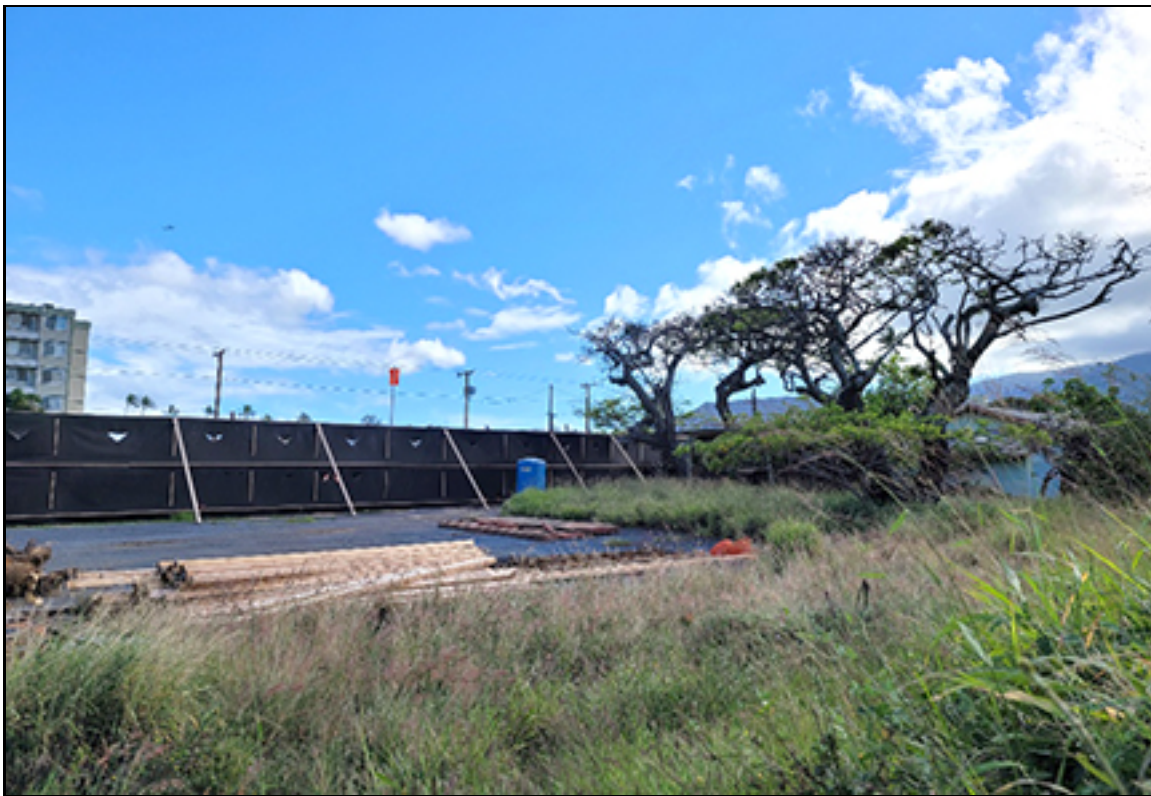
Figure 4. Area of construction disturbance with both graded and adjacent unmaintained ground present.
