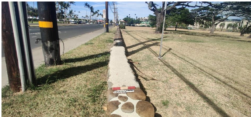
Figure 23. Photo of the northern wall, facing east. Note the repaired section of cement.
