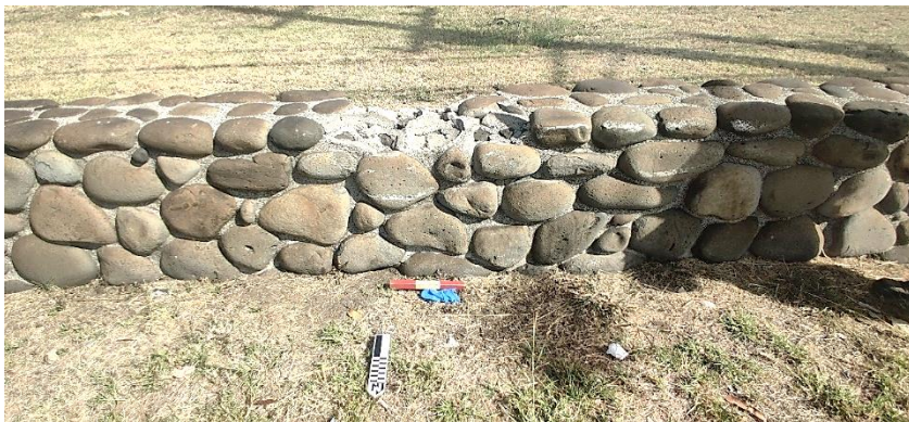
Figure 28. Example of missing stones in the northern wall, facing south.
