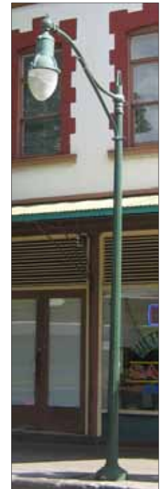
Typical Lighting Standard
