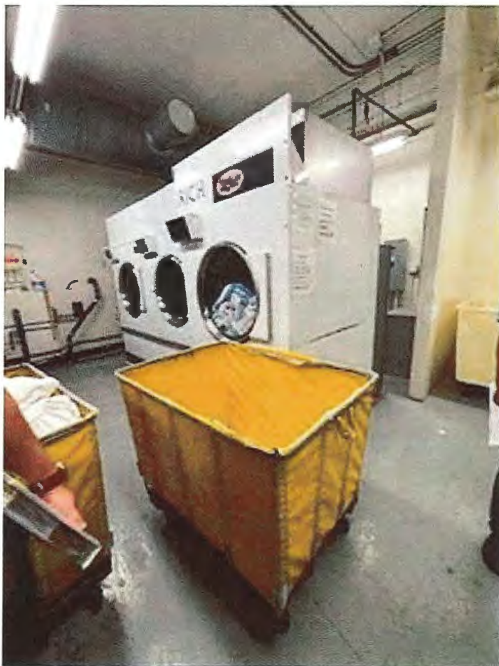
Central Laundry Room
