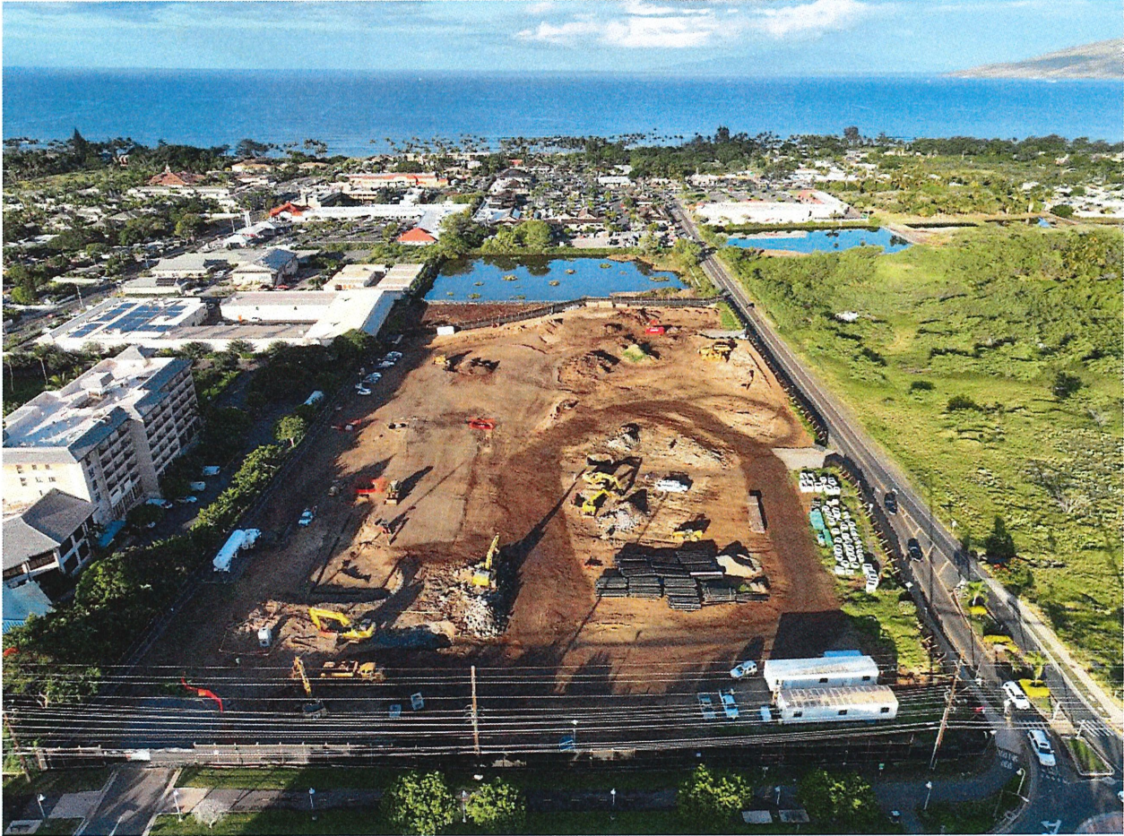
Aerial photo of entire Hale O Pi'ikea project site and ongoing construction with Phase I.
